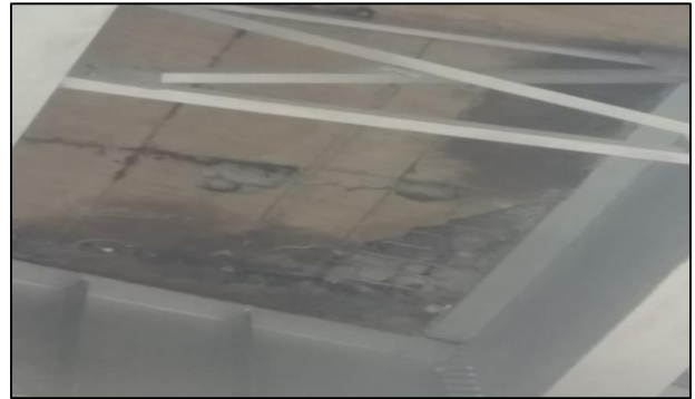
Fig 16. Bottom Side view of Distressed Deck Slab
