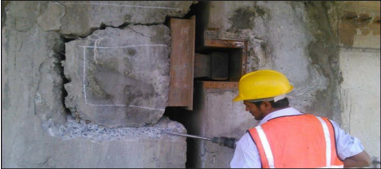
Fig 2. Failed Hinge Connection of Bharuch Bridge
