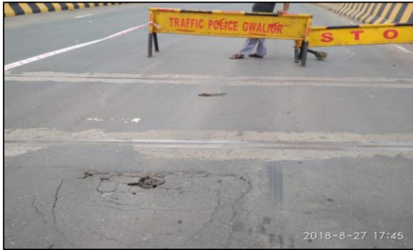
Fig 15. Distress Portion of Deck Slab
