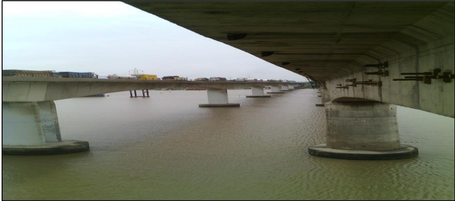
Fig 1. 55-Year-Old Bridge in Bharuch.
